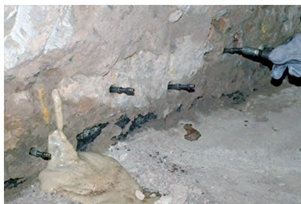
Preliminary injection of a PU injection foam resin into masonry with cavities
