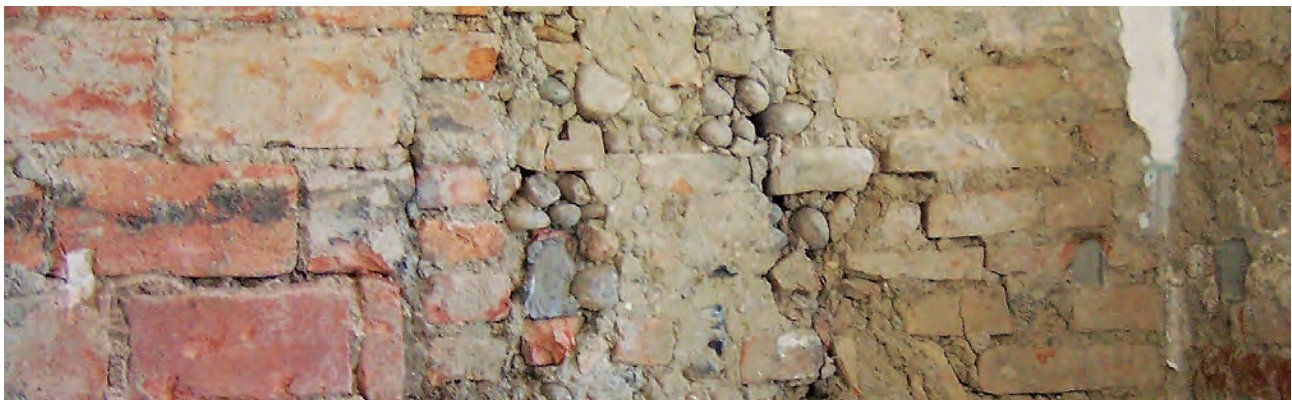
Damages in mixed masonry
