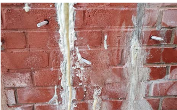
Fig. 5: Injected and filled crack
