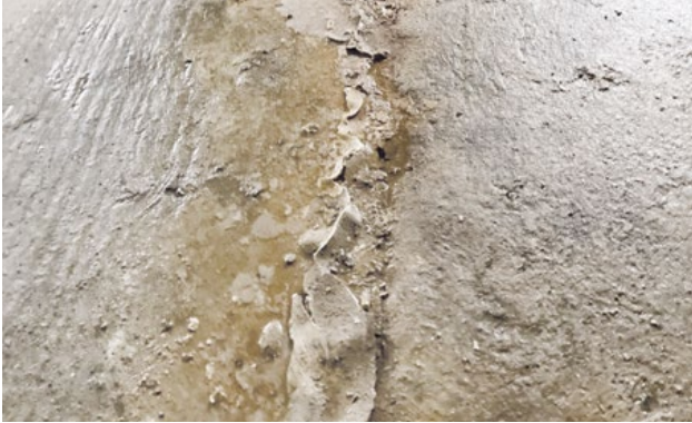
Fig. 1: Actual condition of joint before sealing
