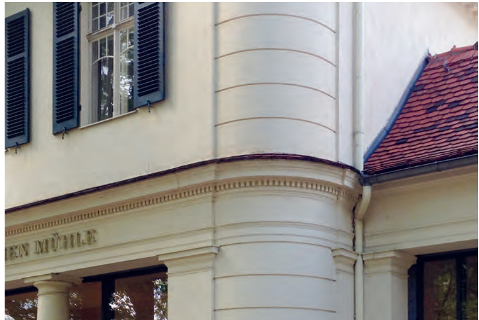
Part of the historical facade coating was provided with a reversible protection
