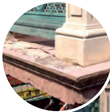
Damages at balcony ceiling
